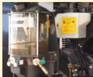
Automatic greasing system
